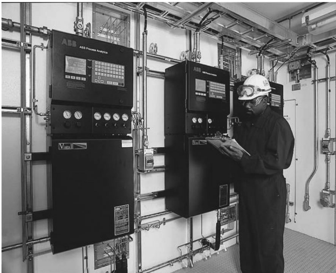
Figure 2-3: An Inside View of an Analyzer Shelter (Courtesy of ABB Process Analytics)
